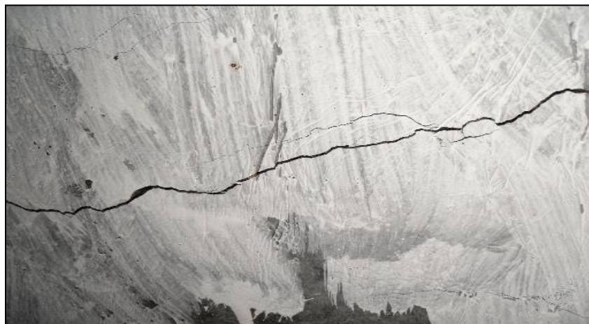
Fig. 6: Failure of Slab at Ultimate Load
