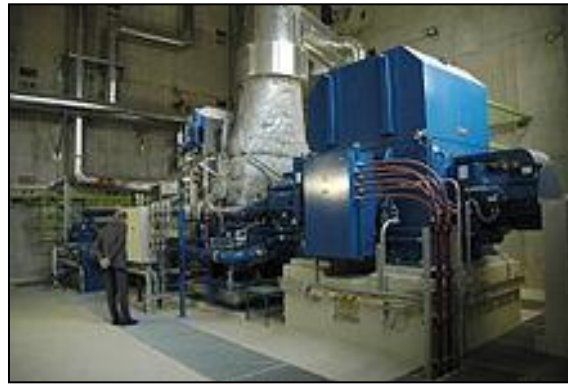
Fig. 4: Steam Turbine Fuelled With Biomass
