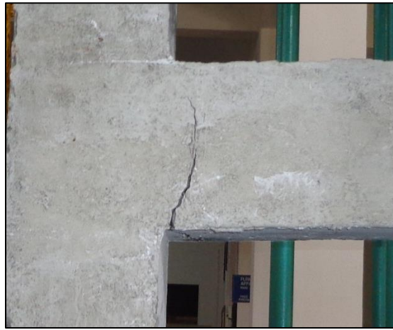
Fig. 6: Failure pattern of SFCC Beam Column Joint
