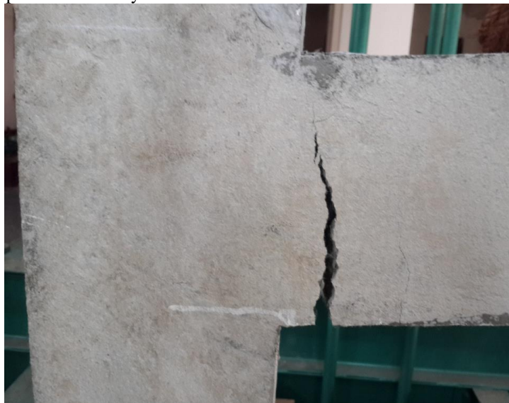
Fig. 5: Failure pattern of PFCC Beam Column Joint
