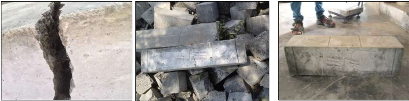
Fig. 8: Flexural Cracks in Beam
