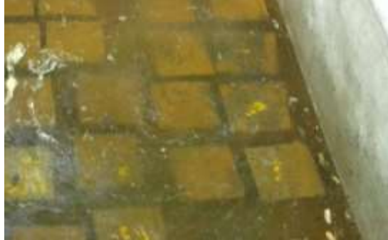
Fig. 4.3: Acid attack on concrete
