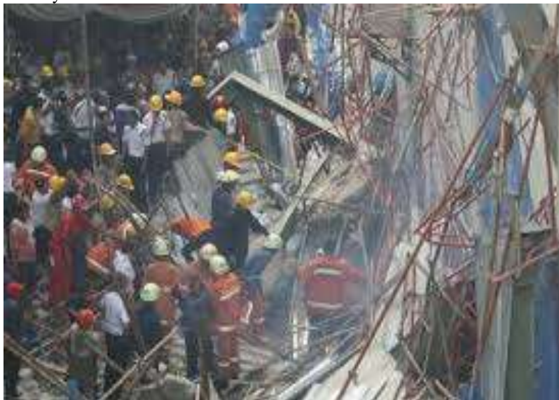
Fig. 1.4: Scaffolding collapse fetal accident [4]
